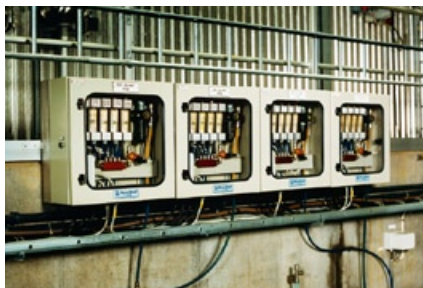
AIR SUPPLY CONTROL PANELS.
